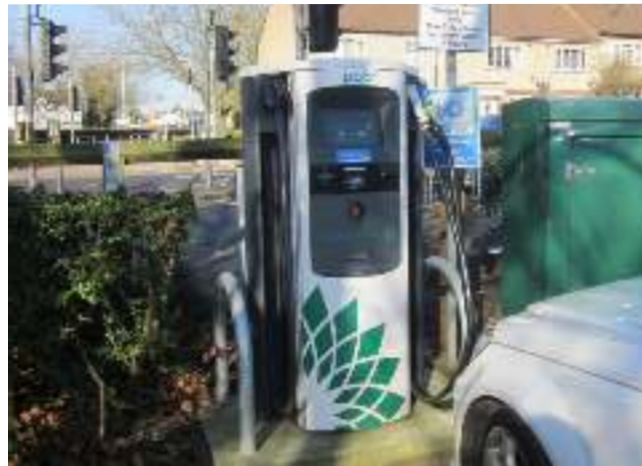
Figure 15. EV charging points
