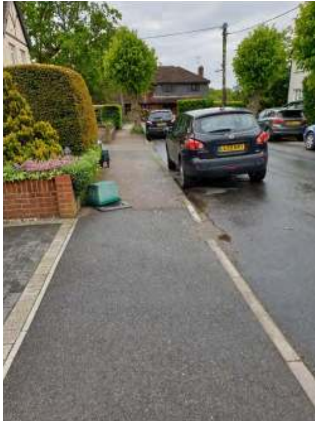
Image 2.6 - Existing Footway Surface - The Avenue
