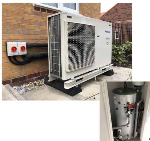
FIGURE 6: HEAT PUMP INSTALLATION
